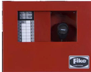
Local Operating Console
