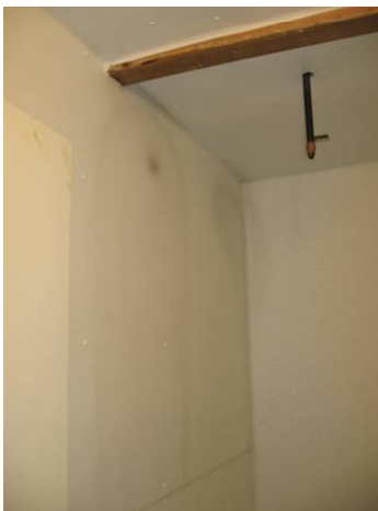
Figure 1: FK-5-1-12 Discharge onto FRP Cladding
